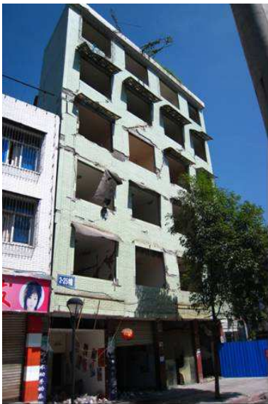
Figure 22. Pounding between two different building in Dujiangyan
