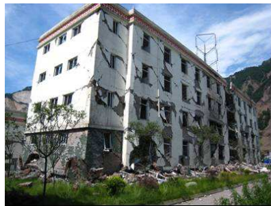
Figure 15. First storey of 5-storeys building in Ying Xiu has totally collapsed.
