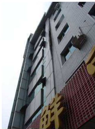
Figure 17. Façade element damage of building in Mianyang.
