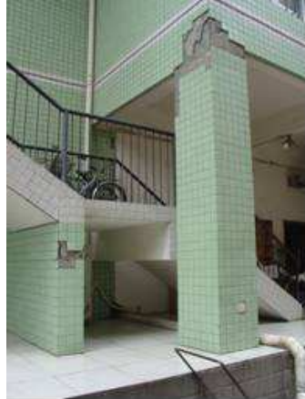
Figure 19. One of building in Mianyang suffered from beam-column joint failure
