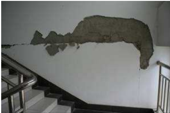
Figure 7. Horizontal crack at the Sichuan University office in Chengdu.
