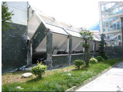
Figure 14. Building in Ying Xiu collapsed because of soft storey mechanism on one direction and short column on other directions.
