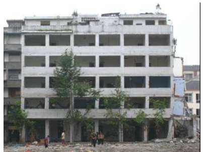
Figure 16. Soft storey damage of second storey with drift about 5.6% in Dujiangyan
