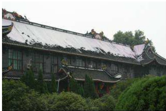
Figure 10. Many old buildings at Sichuan University in Chengdu suffered from roof tile damage.
