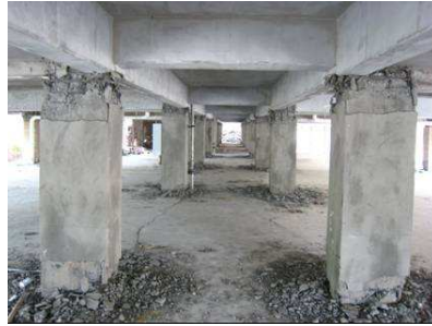
Figure 12. Plastic hinge failure at all first-storey columns of Figure 11.
