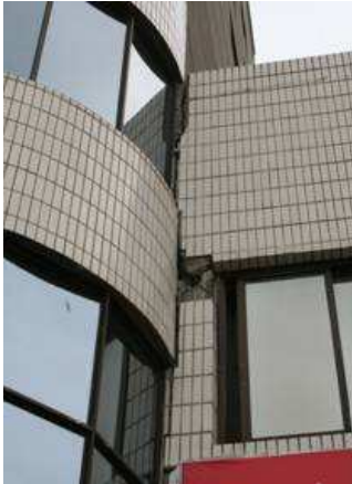
Figure 18. Column shear failure at one of building in Mianyang.
