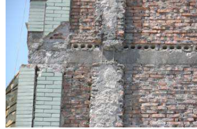
Figure 20. Poor beam-joint connection
