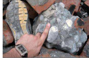
Figure 21. Bad gradation of aggregates.
