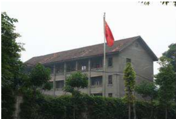
Figure 9. A building in Chengdu with roof tile sliding.
