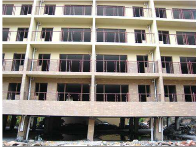
Figure 11. Soft first storey of 6-storeys building in Dujiangyan with drift about 7.5%
