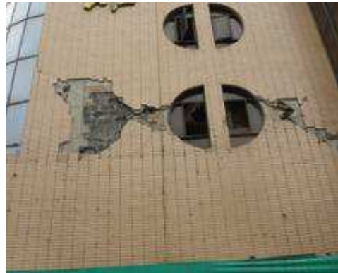
Figure 8. Diagonal shear crack of one of the buildings in Mianyang.
